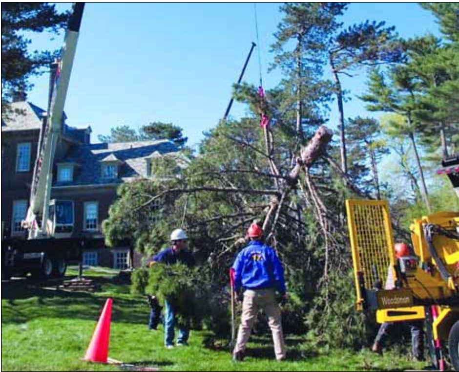
One of two 120-foot cranes owned and operated by Maltby & Co. of Stoughton, Mass., a TCIA member company, removes a tree at the Crane Estate in Ipswich, Mass. The company mostly uses cranes for removals, but will also sometimes use its cranes for planting.
