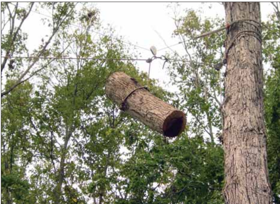
A log has been hauled into the air and is ready to be lowered on the speed line.
