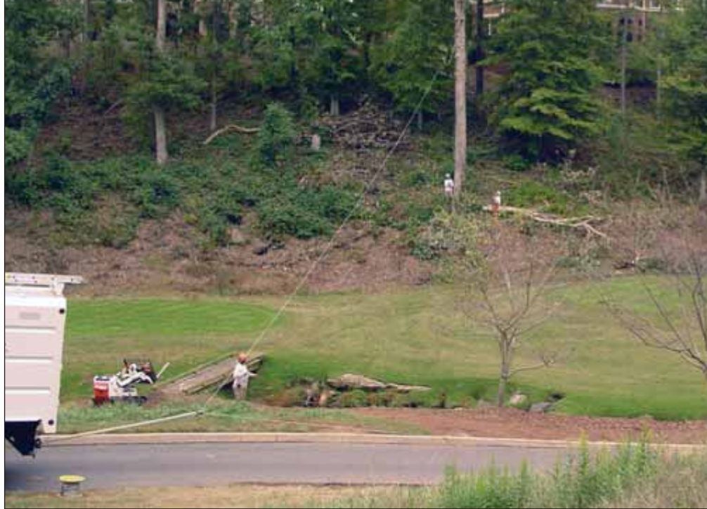
Looking across the cart path, stream and tees to the hillside where the storm damage occurred. The pickup used to tension the speed line is just out of view on the right on the cart path. The pull line has been reset and is slack.
